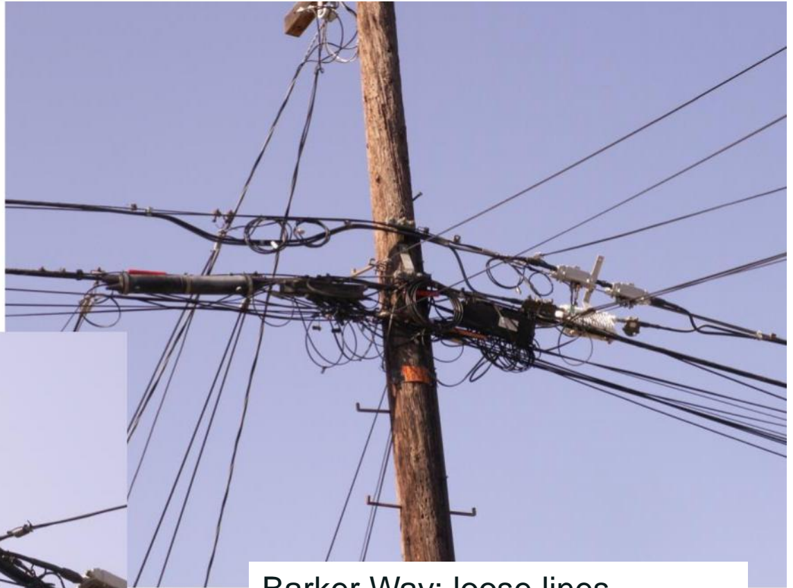
Barker Way: loose lines, inadequate spacing; exposed connectors
