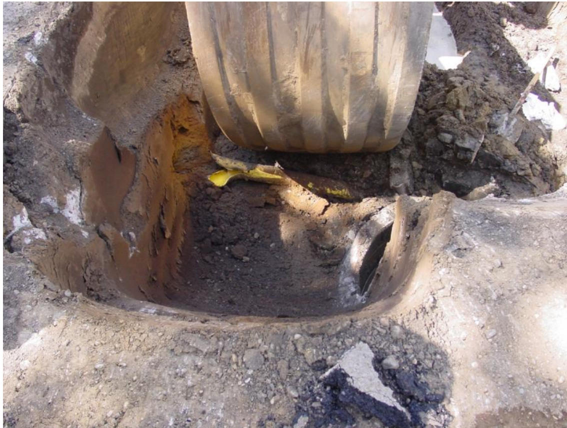
Backhoe strikes buried gas pipeline.
