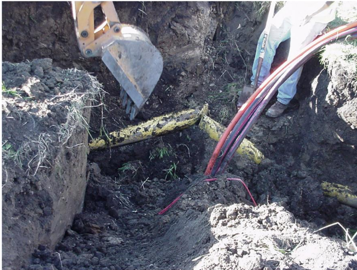
Backhoe strikes and damages gas pipeline.
