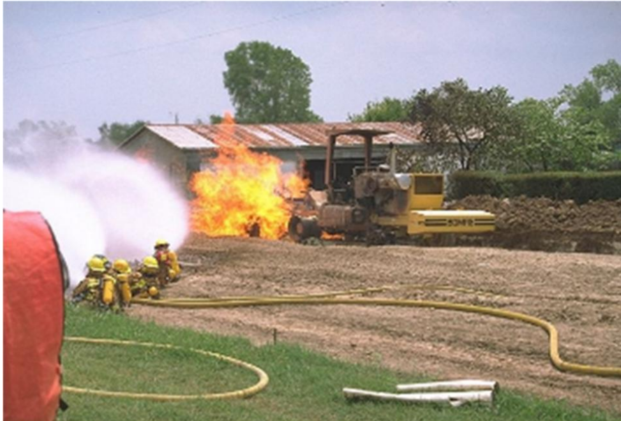
Excavation hits a gas pipeline and causes a fire in a farm field.
