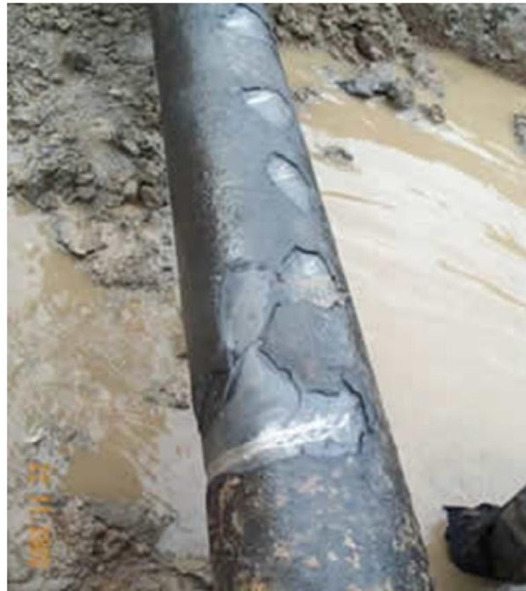
Pipeline with excavation damage.
