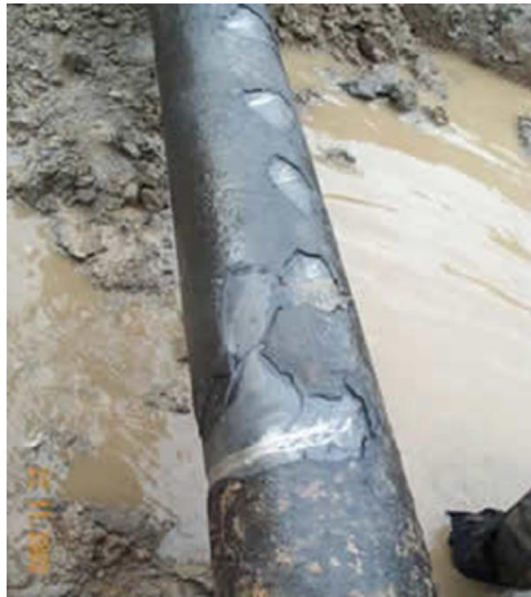
Pipeline with excavation damage.
