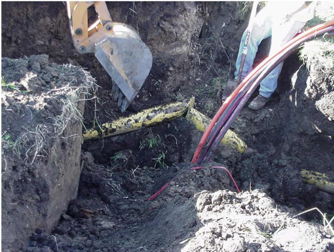
Backhoe strikes and damages gas pipeline.
