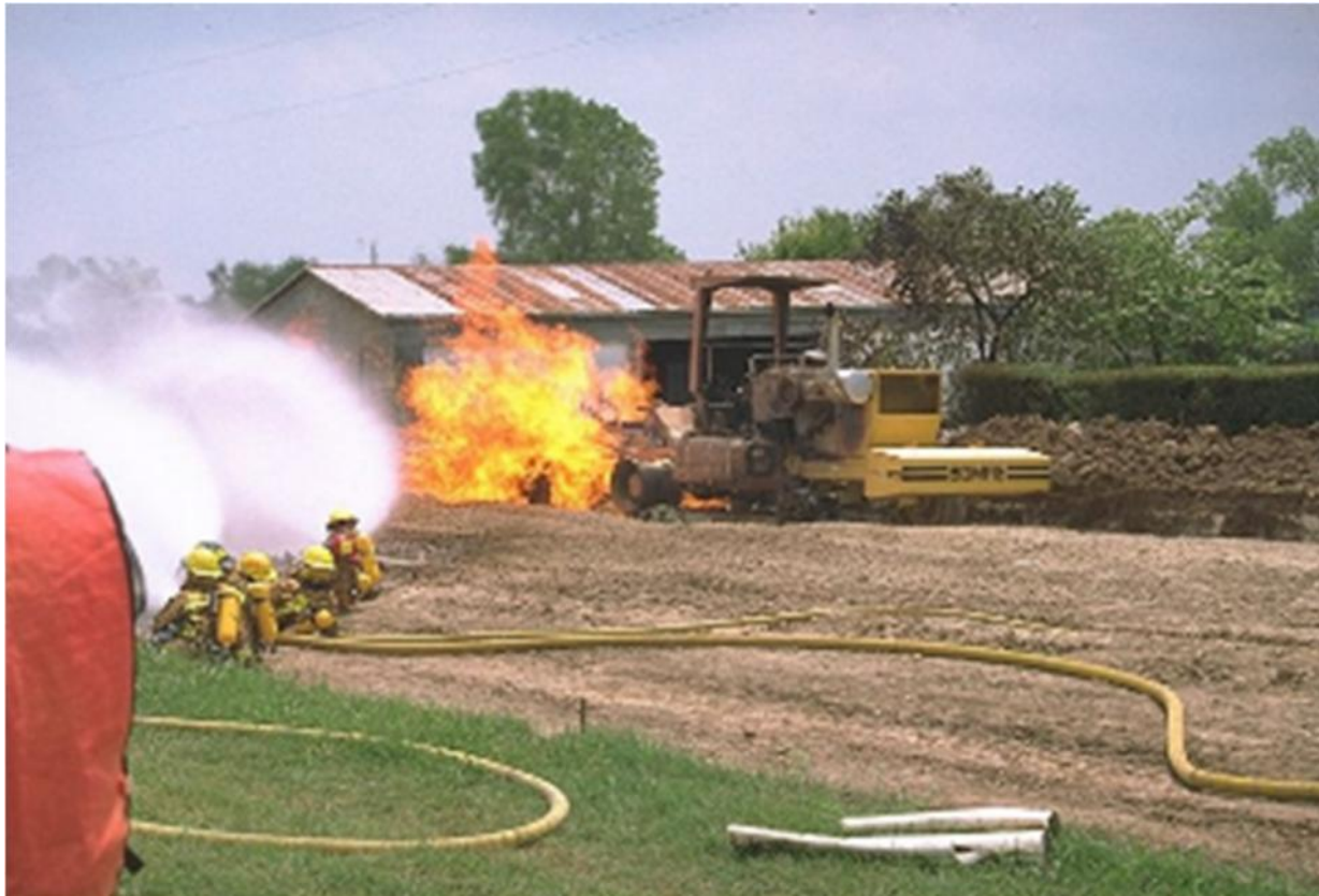
Excavation hits a gas pipeline and causes a fire in a farm field.
