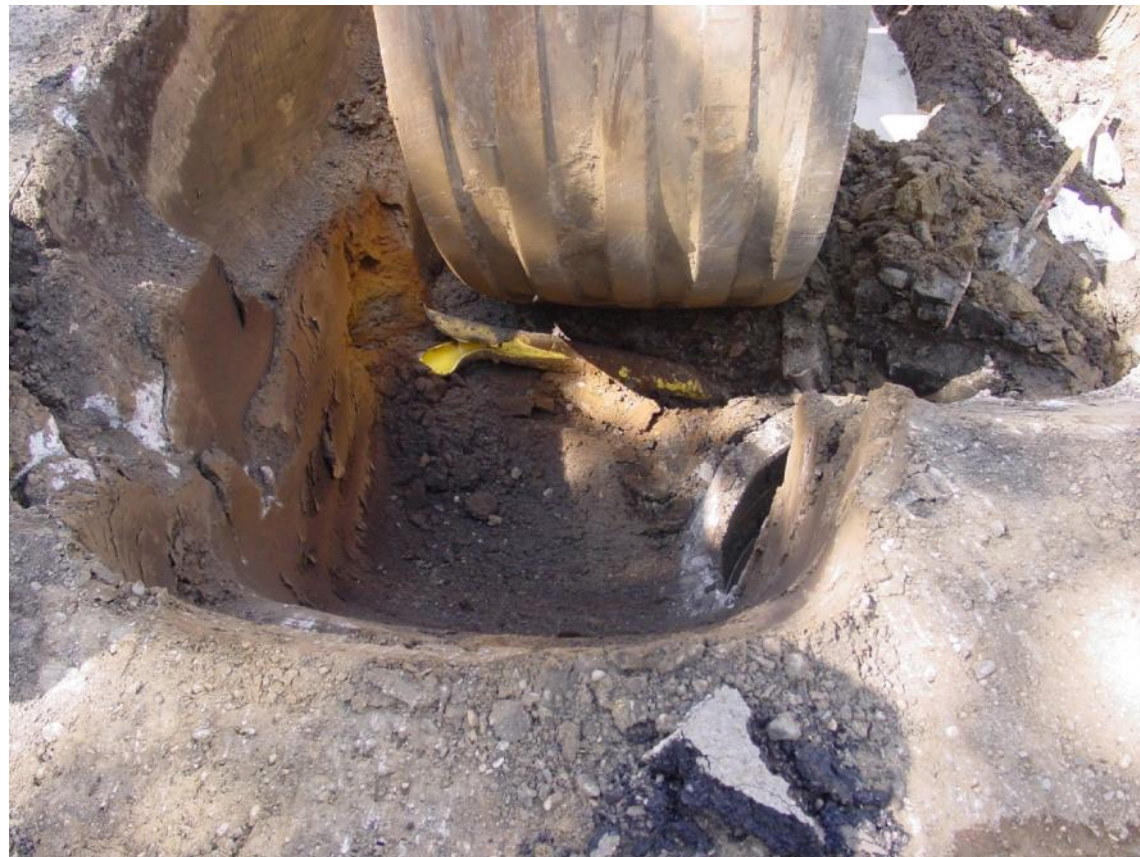
Backhoe strikes buried gas pipeline.
