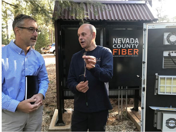
Figure 6: "Fiber in the Forest", Nevada County Fiber Inc. demonstrates to the Rural County Representatives of California, the Central Data Center and underground & fire safe deployment of 25 underground FTTH connections in one of rural Nevada County's most challenging build areas.
