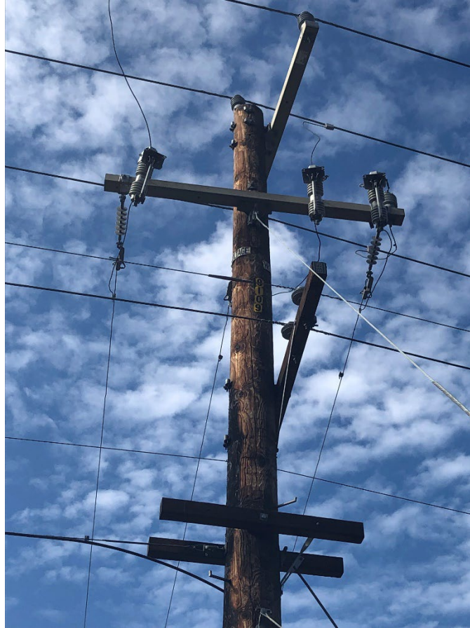
Figure 1: Incident pole, showing burn damage from the fire.
