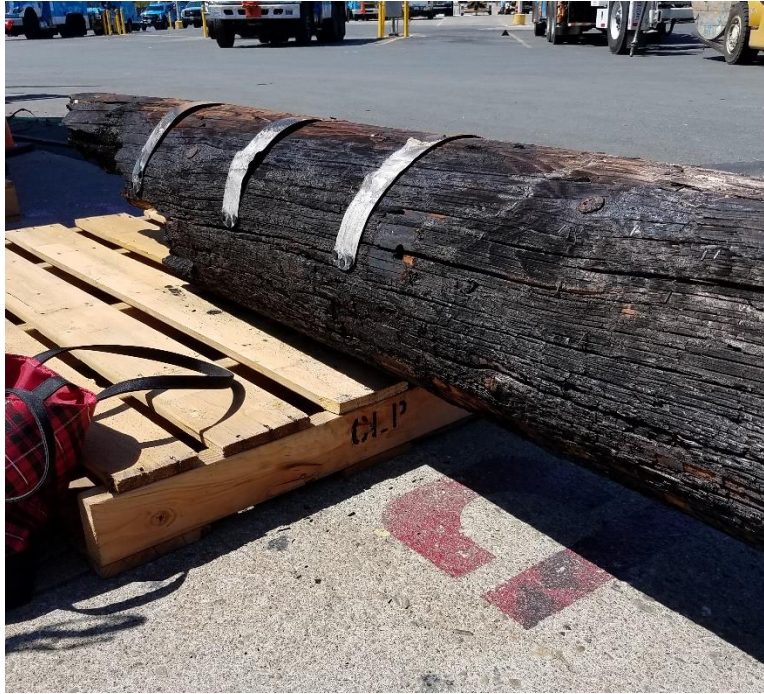
Figure 1: Segment of Pole 1. This appears to be the point of failure.
