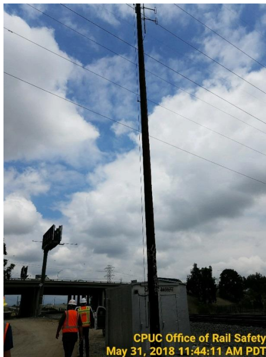
A CPUC inspector observed a UPRR PTC wayside installation and associated PTC radio equipment. PTC antennas are shown on the top of the pole.
