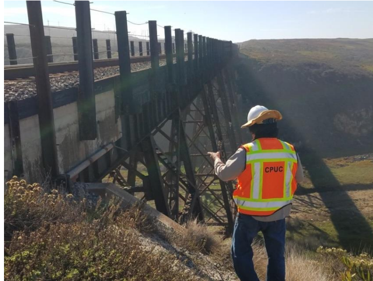
CPUC railroad safety bridge inspector looking over ballast deck bridge substructure for structural integrity and associated potential risks
