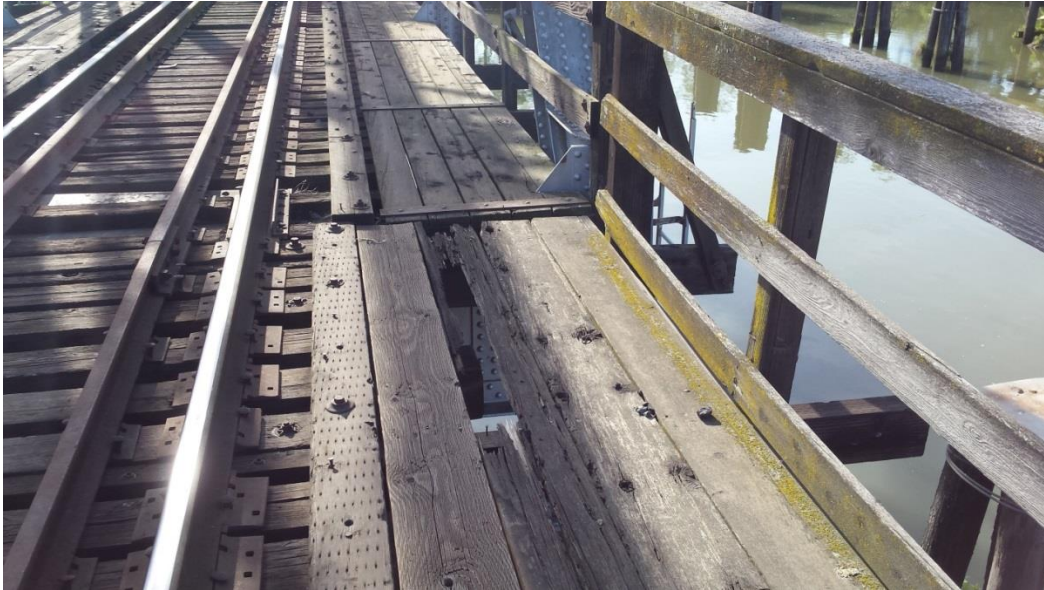
Unsafe walkway on the San Joaquin River Bridge
