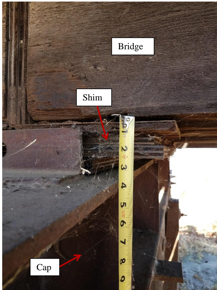
Deteriorating shims compounding out of level condition under bridge
