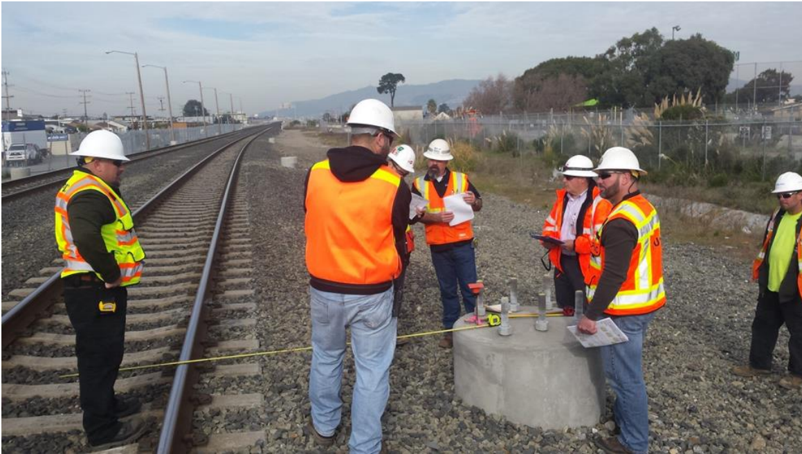
CPUC and Caltrain personnel inspecting in San Bruno at one of the new foundations that will support the upcoming electrification
