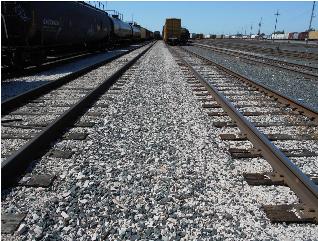
Oversized ballast location after large ballast removal; replaced with ballast complying with GO 118-A.
