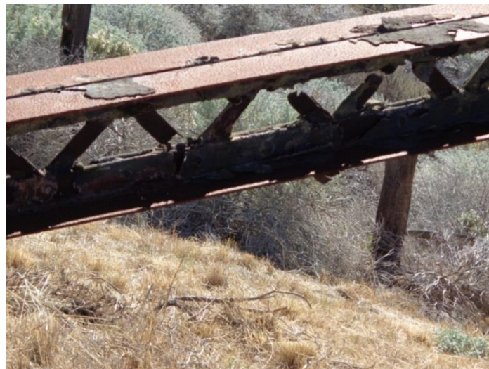
Deteriorated steel on a UPRR bridge, Vandenberg Air Force Base
