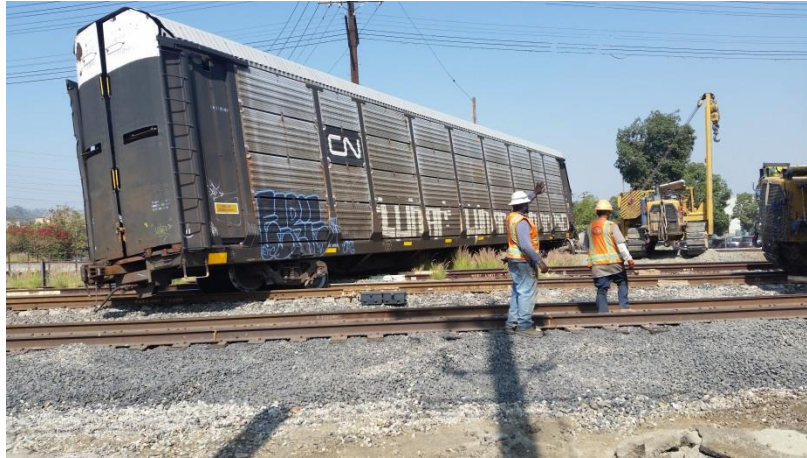
Derailed auto rack train car
