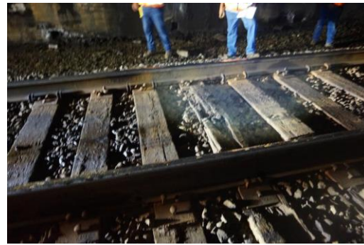
Loose spikes found in tunnel 33
