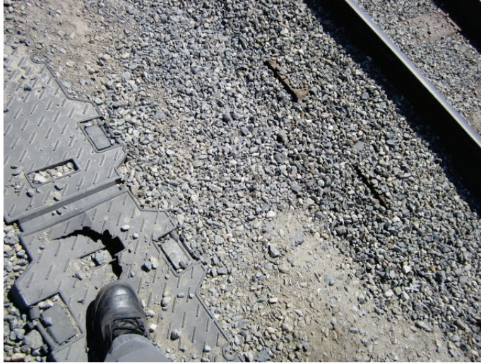
Broken plastic covers intended to protect workers from tripping and falling into an underground cavity that houses an assortment of cables
