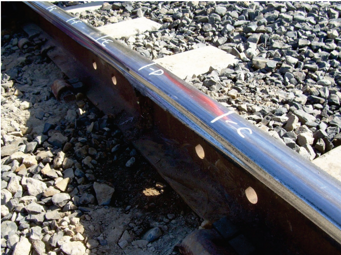
Insulated joint plug weld near point of derailment
