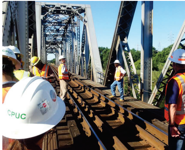
Risk Assessment Section and ROSB personnel on a Union Pacific Railroad bridge in Sacramento, California during a bridge inspection.
