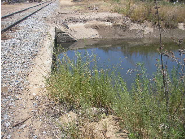
Initial inspection: faulty walkway, no handrails
