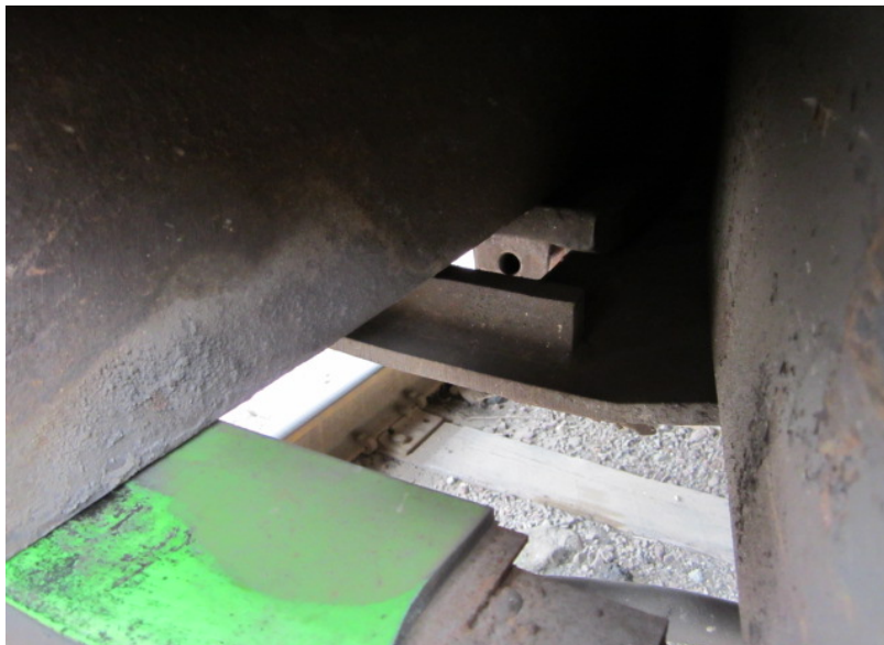
This photo shows the hole where the end of the bolt should be.
