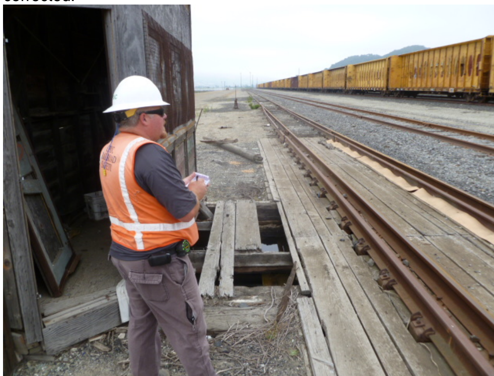
Hazardous walkway condition at UPRR's Watsonville Yard
