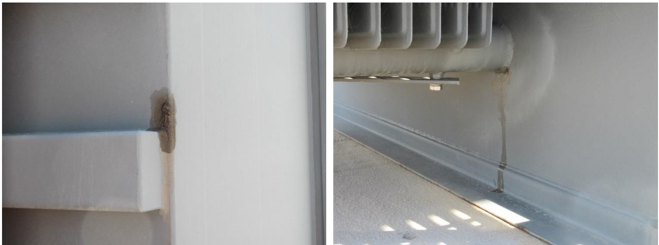
Figure 3 & 4: Pinhole Oil Leaks from Transformers next to Inverter B8-09 and B18-06.
