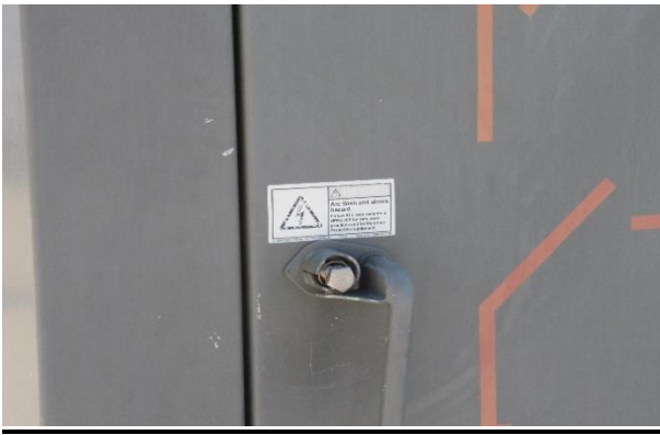
Figure 12: 07- PVCS Switch Cabinet
