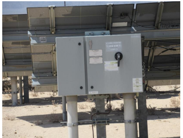
Figure 2: Faded signs/labels on the combiner boxes
