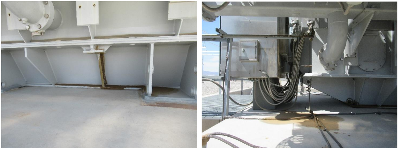
Figure 7 & 8: Oils Leaks on Transformer GSU2 in substation.
