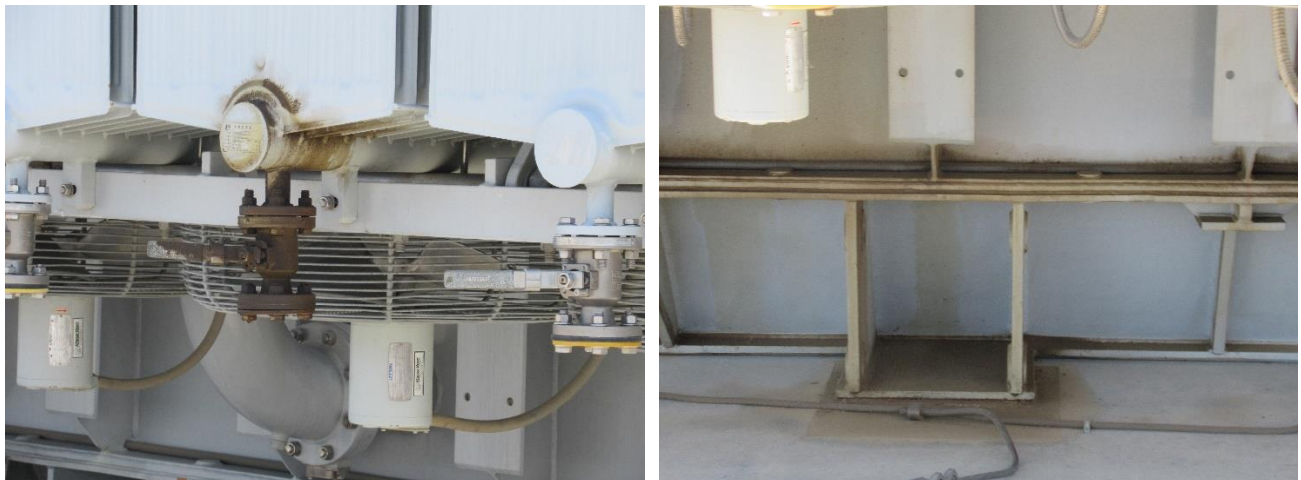
Figure 5 & 6: Oils Leaks on Transformer GSU1 in substation.
