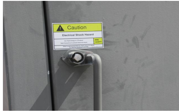
Figure 13: 18-PVCS Switch Cabinet
