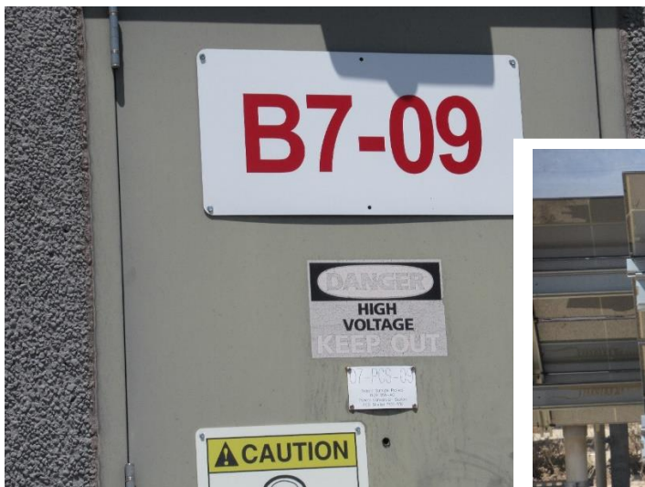
Figure 1: Faded High Voltage Sign on inverter facility door.
