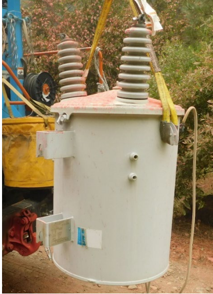
Figure 6: Transformer from pole 435.
