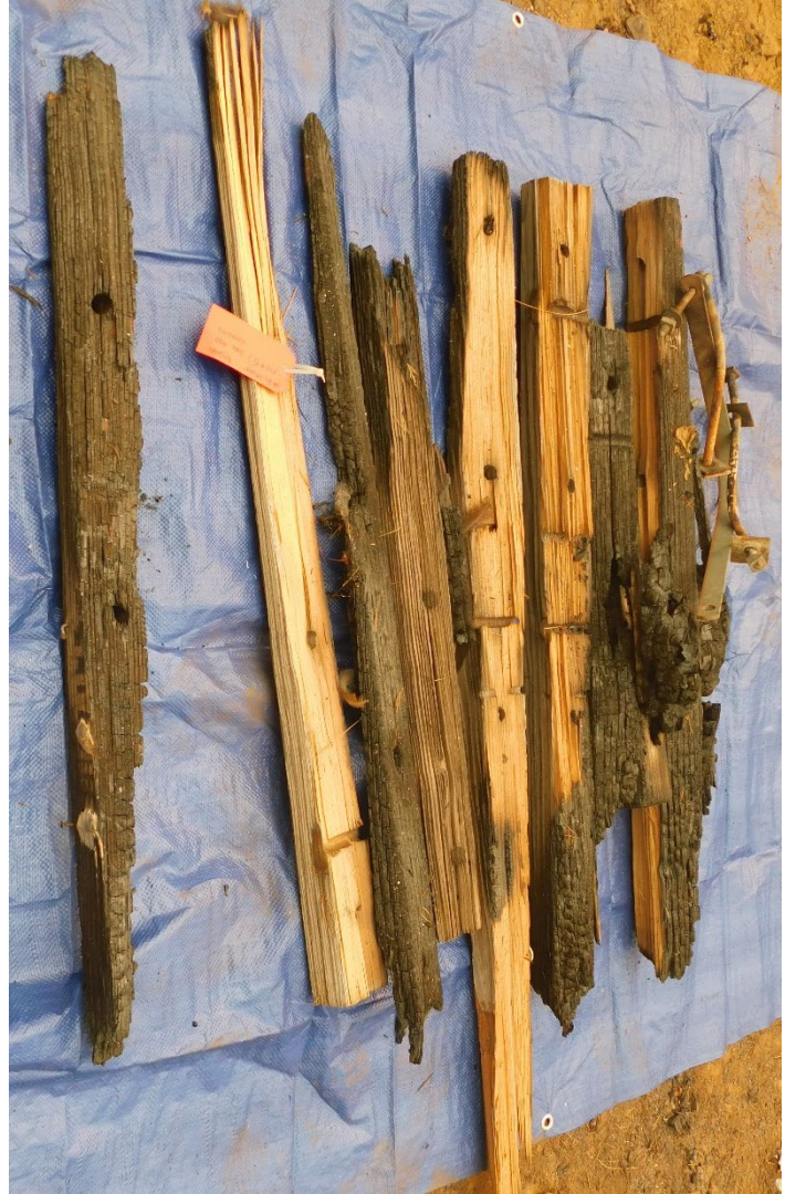
Figure 11: Crossarm remains from base of pole 433.
