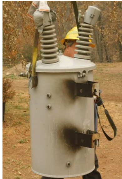
Figure 9: Transformer from pole 432.
