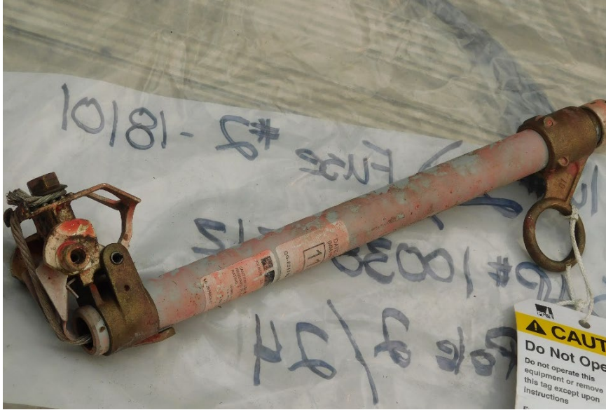
Figure 4: Second fuse does not appear to have blown.
