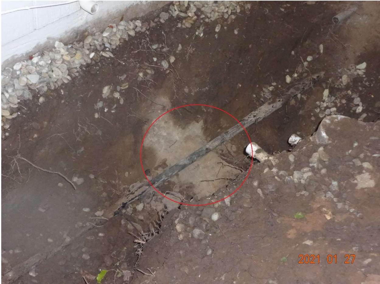
Figure 4: Excavated trench next to the house with 3/4-inch gas service line and sewer lateral. The red circle highlights where the two pipes are in contact. The soil near the intersection of the pipes was dry, although most of the soil brought up from the pit was wet.
