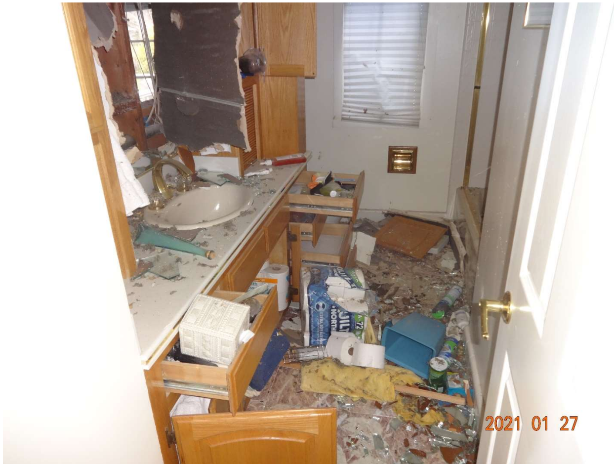
Figure 3: The damage to the North bathroom. The sheetrock and insulation had blown out from the wall. The wall mirror and the sliding glass doors around the tub were shattered.
