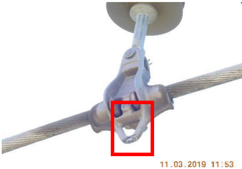
Figure 1: The damaged insulator, burning mark on the pole and cables (marked red)
