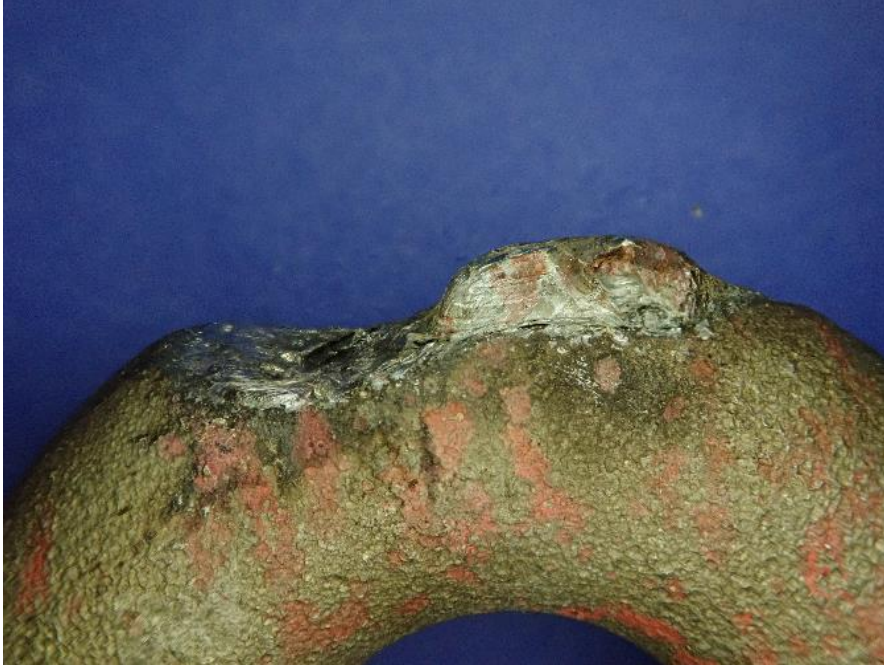
Figure 2: The damaged insulator shoe (suspension clamp) 1
