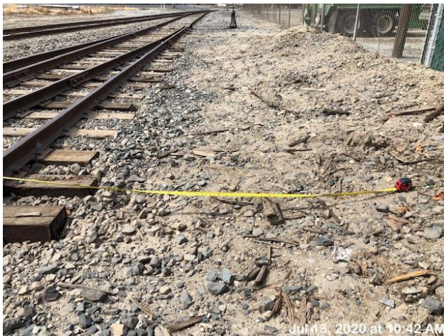
Before: Irregular walkway surface
