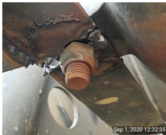
RSD Mechanical inspector discovered the air reservoir tank mounting brackets were broken and not properly repaired. The train brakes on this rail car may become ineffective due to this defective condition.
