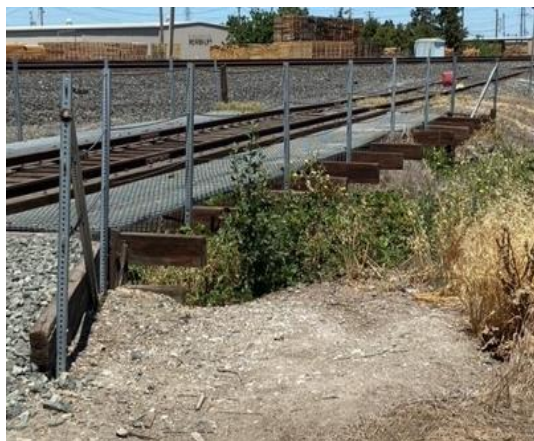
Before: Vegetation growing around the bridge
