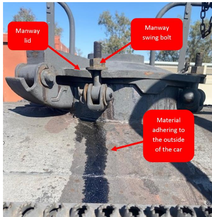
Manway on top of tank car with residue adhering to outside of car
