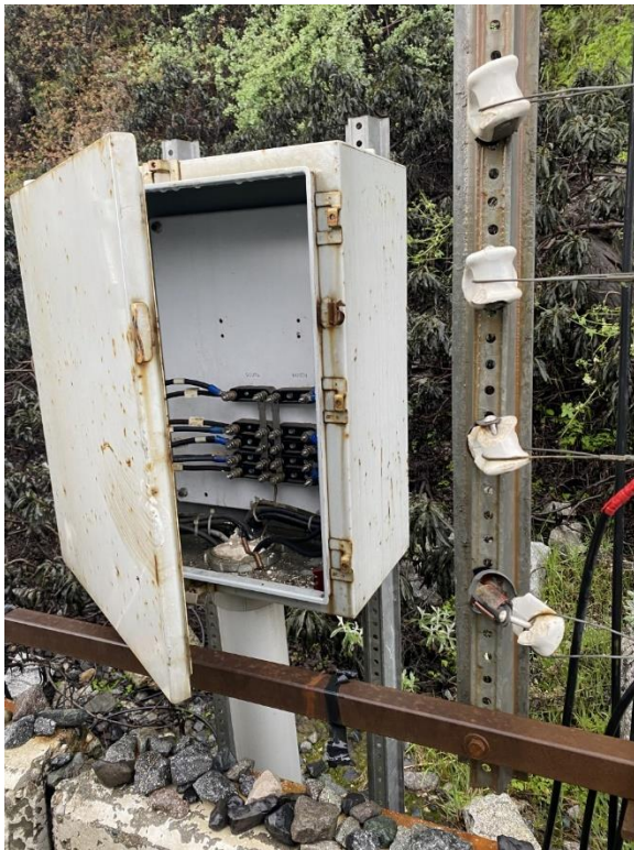
Unsecured junction box
