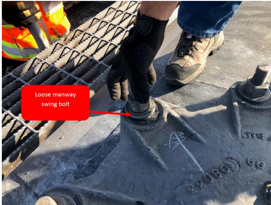
One of five loose manway swing bolts
