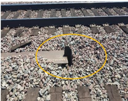
Uneven walkway with obstruction on bridge deck
