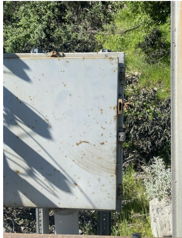
Junction box secured
