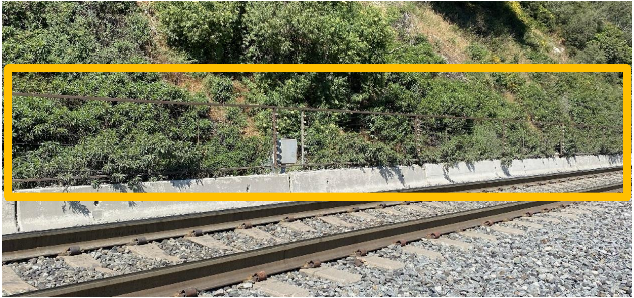
Slide fence provides warning if debris fall from the hill onto the right of way
