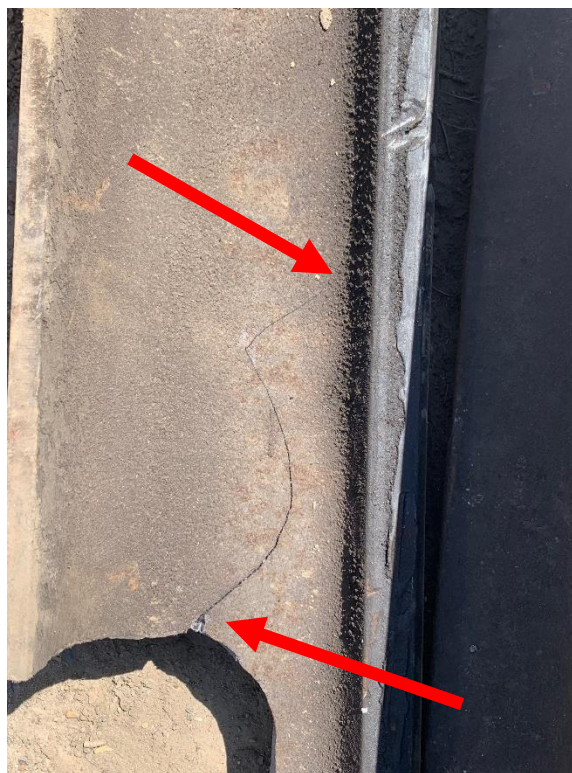
8-inch crack in the rail extending up to the head of the rail
