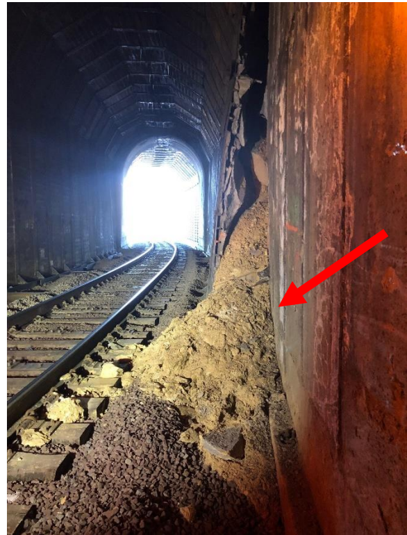
Break in wall, BNSF tunnel
