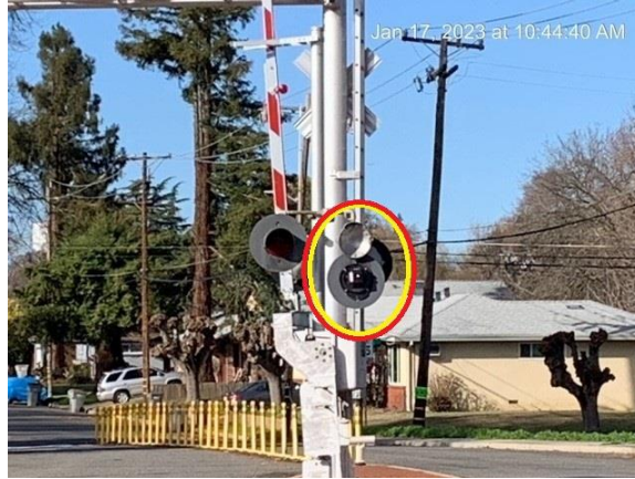
Signal light hanging from the housing structure
