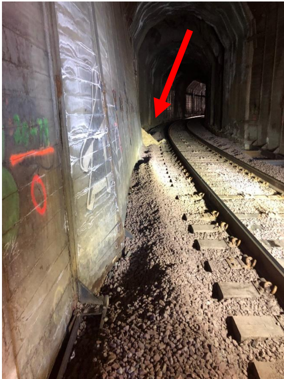
Shift in wall, BNSF tunnel
