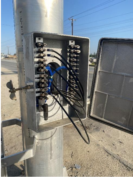
Before: Unsecured Junction box
