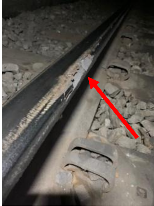
Degraded rail section
