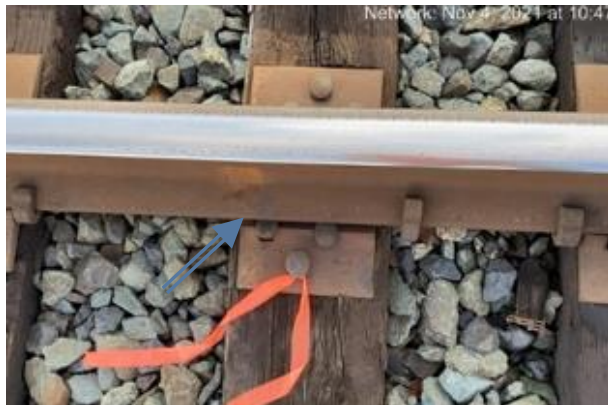
Before: Spikes between the tie plate and rail base
