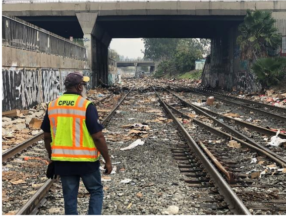
Before: Walkways covered by debris
