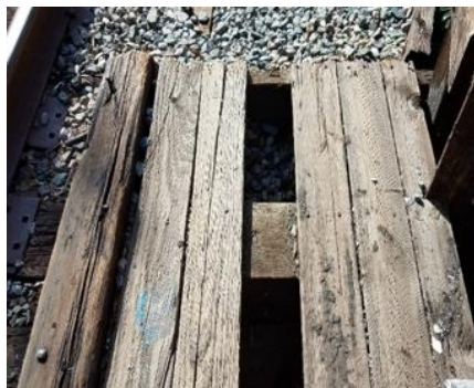
Before: Walkway plank missing on bridge deck
