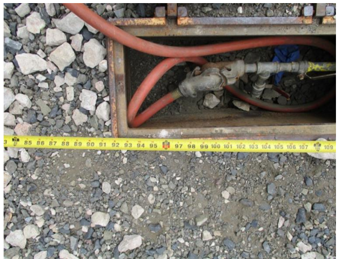
Before: Detail, open air charging box
