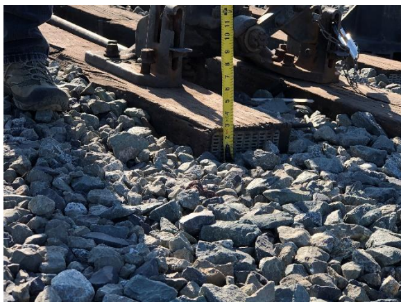
Before: Exposed railroad ties near track switch
