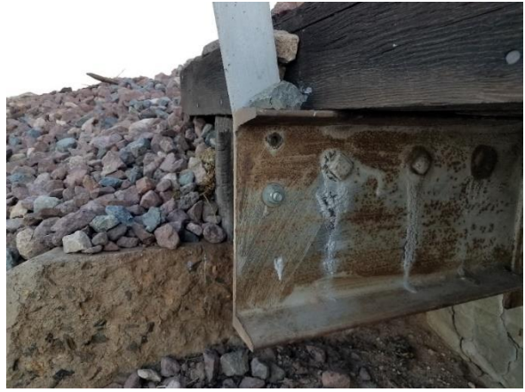
Before: One of six missing bolts
