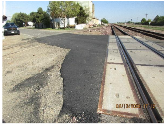
After: Le Grand St. crossing brought into compliance
