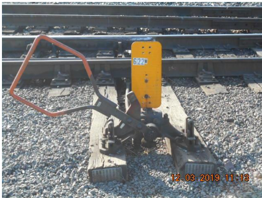
Before: Ballast around switch is below the top of the ties, creating tripping hazard
