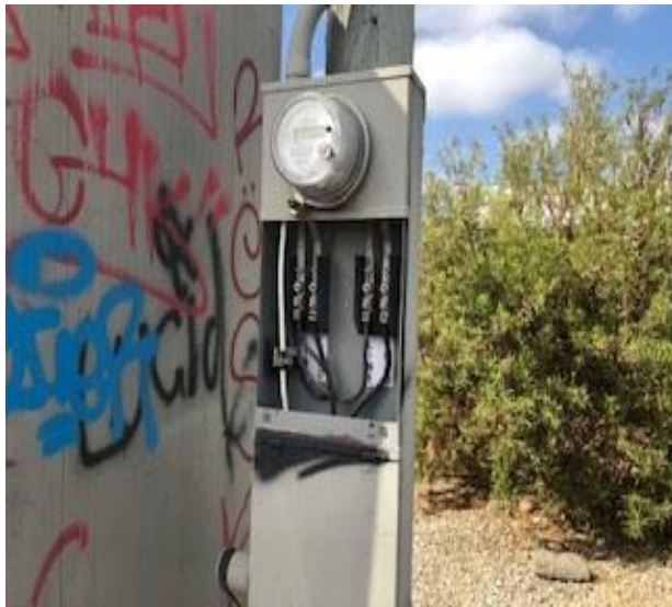
Before: Vandalized power supply box
