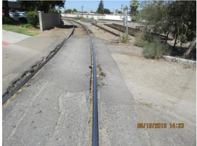
Before: Degraded asphalt at crossing
