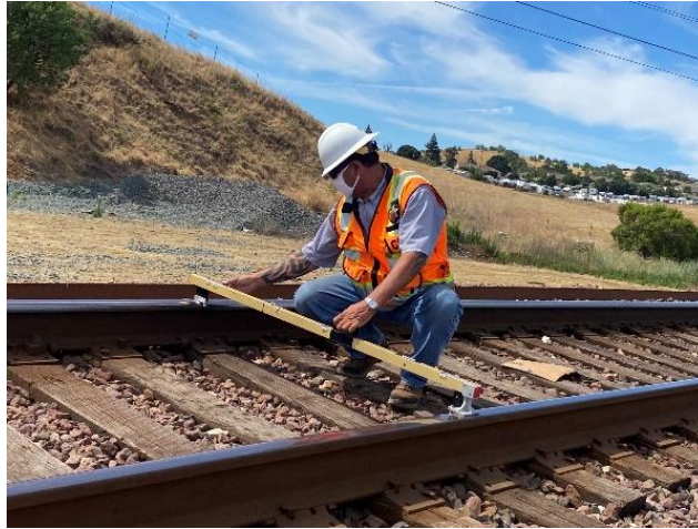
RSD inspector wearing mask, measuring main line track with a level during an inspection
