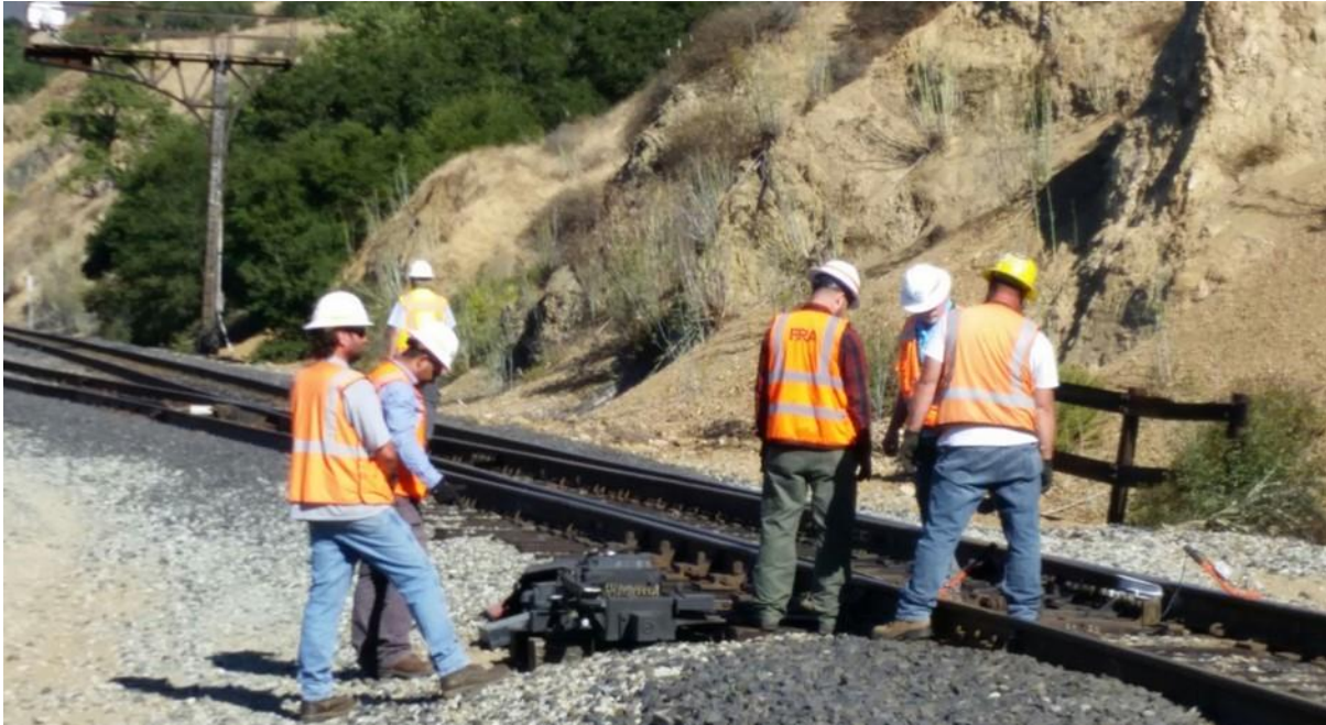
RSD and FRA Signal inspectors along with railroad company personnel conducting an inspection of a mainline power switch
