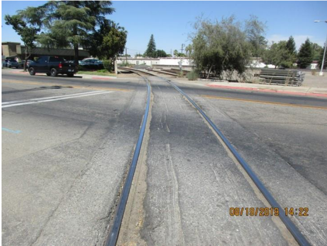
Before: Degraded asphalt at crossing
