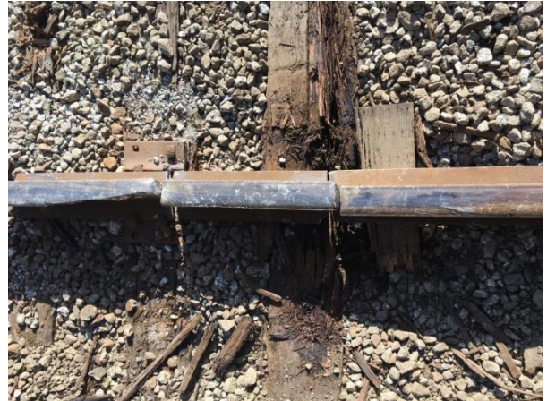
Broken rail, Emeryville
