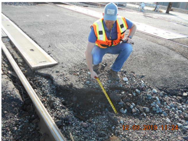
Before: Approach grade exceeds six percent; not in compliance with GO 72-B
