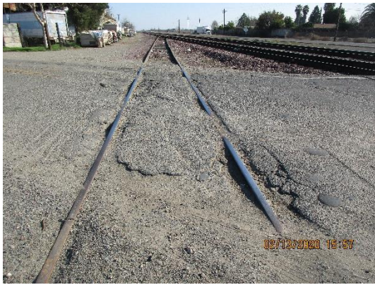
Before: Unsafe conditions at Le Grand St. crossing
