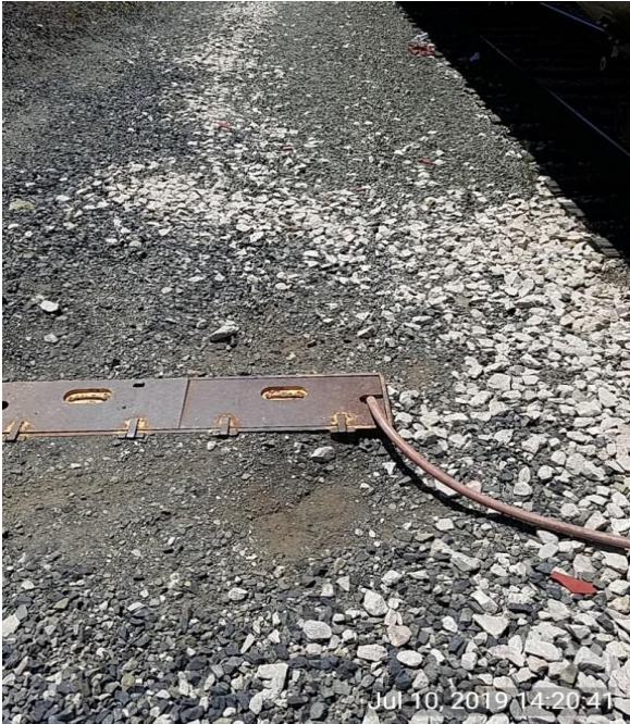
After: Air charging station lids closed
