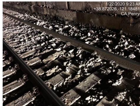
Before: Ballast dislodged due to mud & silt buildup
