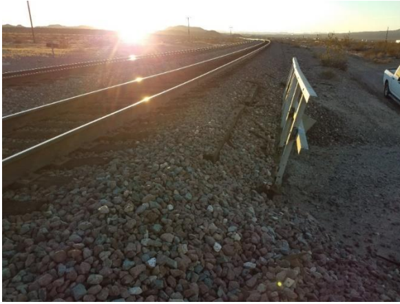
Before: Handrail not in upright position
