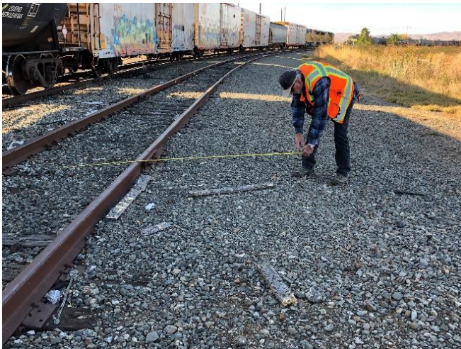
Before: RSD inspector measuring edge of walkway at 8'-6" from centerline of track and noting debris in walkway
