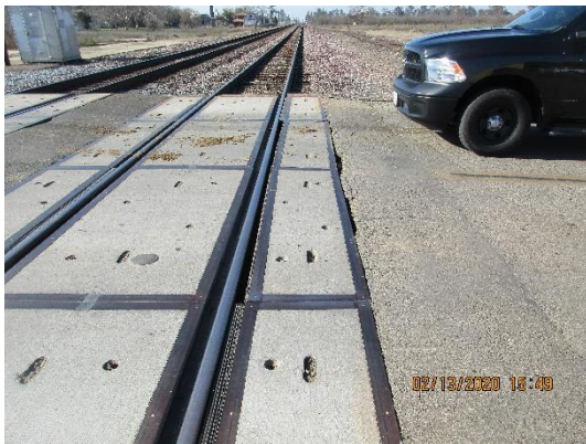
Before: Unsafe conditions at Jefferson St. crossing
