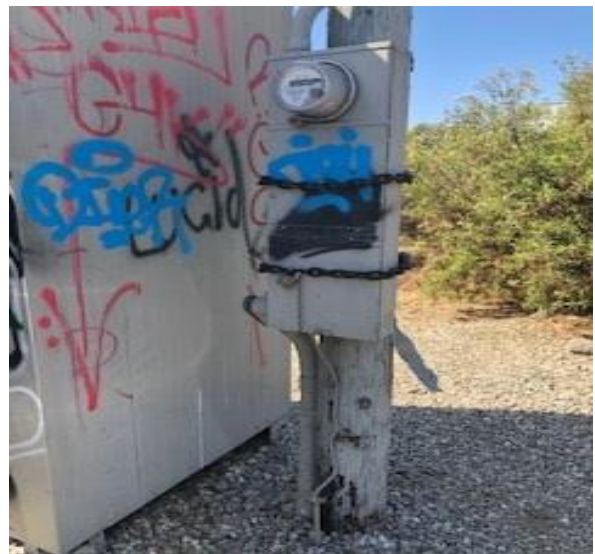
After: Power supply box secured with chain and lock
