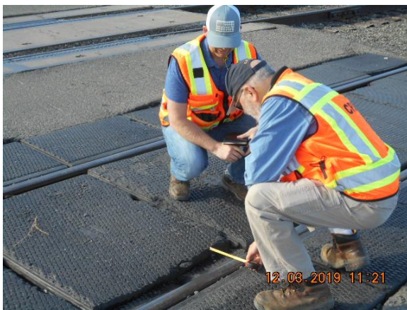
Before: RSD inspectors measuring flangeway gap; gap non-compliant with GO 72-B
