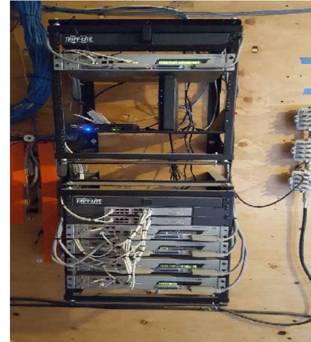
CASF Public Housing Account project Housing Authority of the County of Kern – Green Gardens Main Distribution Frame room
