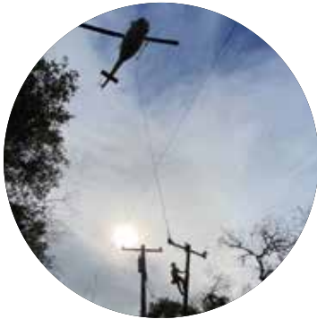
Alvah Group, Inc.: Electric Distribution
