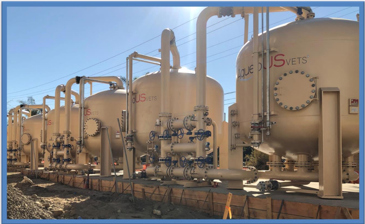
PFAS Treatment System located at San Gabriel's Plant No. 2.
